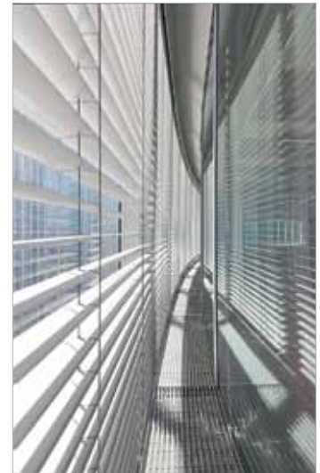
Speciality Venetian Blinds in double skin facade - No. 1 Bligh St, Sydney.
